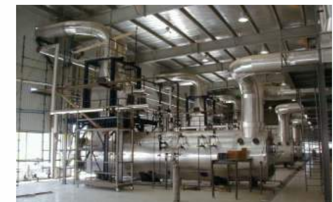
Waste Heat Recovery for Fire tube type for Engine exhaust
